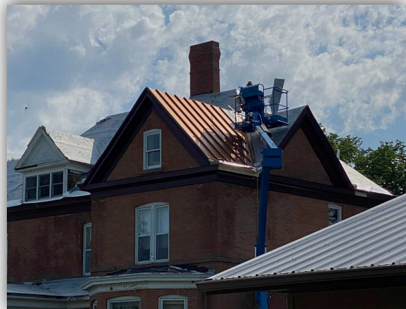
The new Sheffield Metal roof is being installed on the Plummer House in this photo from June 14, 2022. The metal roof is in line with the original design from 1897.
